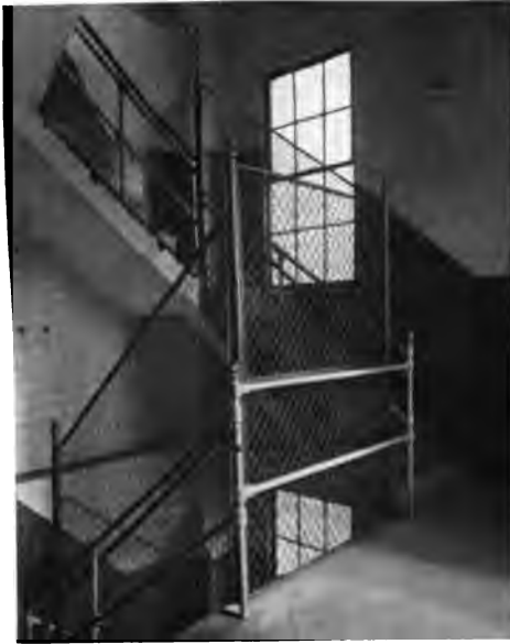
Fig. 1. Railing, etc., at Stairway.*
